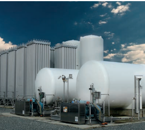
We enable safe handling of cryogenic technical gases and LNG applications
